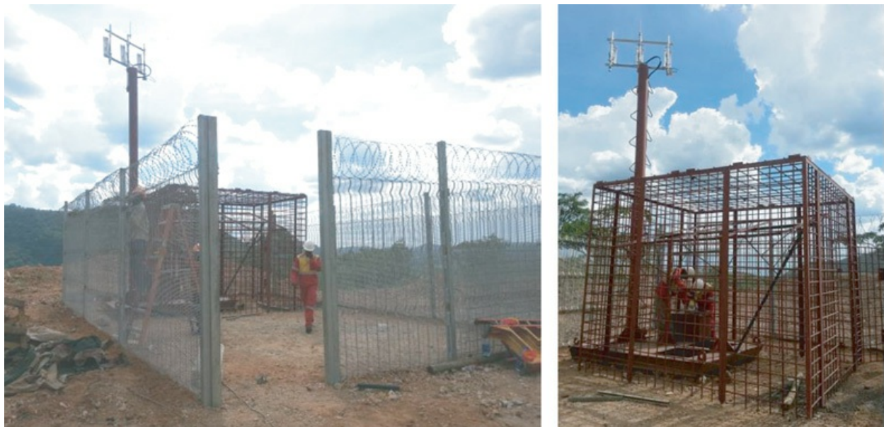
Figure 14-12 Physical Security Protecting Wireless Mesh Equipment at a Mine Site
