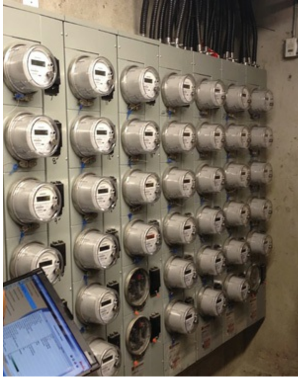
Figure 11-16 A Subterranean Meter Farm in an Apartment Building
