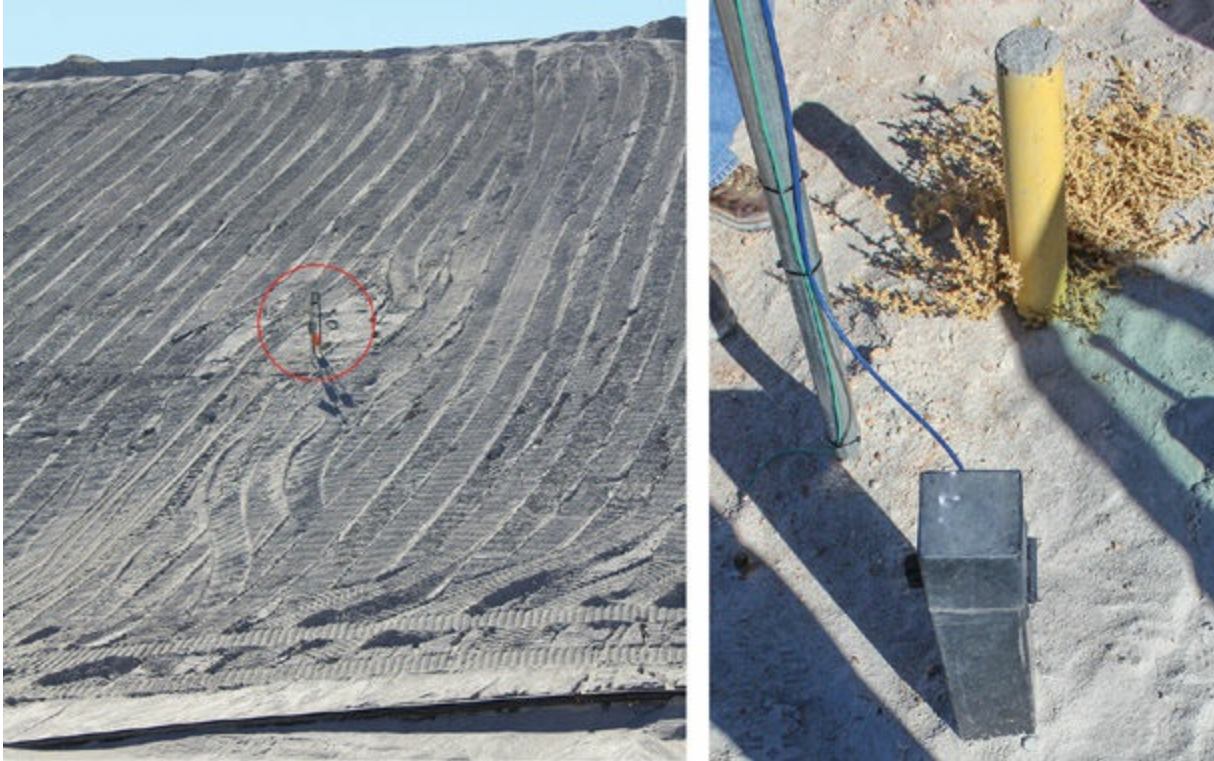
Figure 14-11 A Tailing Pond Earthen Dam with Sensor (Left) and Close-up View of Piezo Ground Monitoring Sensors (Right)
